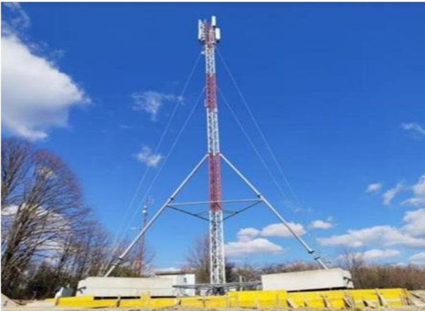
Figure 4.74. Exterior of the base station
